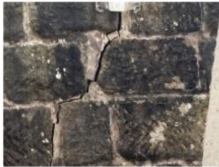
4.) Additional photograph showing the wall crack monitoring, taken from Stoney Lane.
