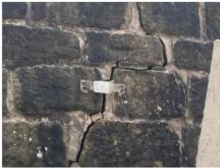
3.) Photograph showing the wall crack monitoring, taken from Stoney Lane.
